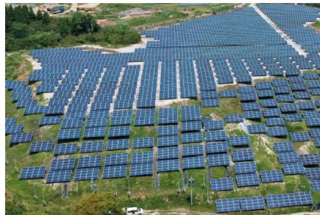
VALORS inc.'s project Kunisaki Solar Power Plant (Kunisaki City, Oita Pref.)
